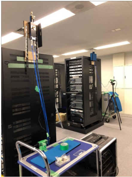
Data center measurement photo
