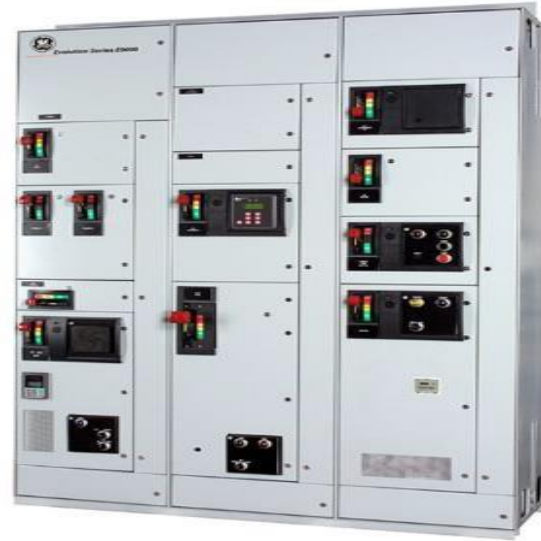
Non-arc resistant LV motor control
