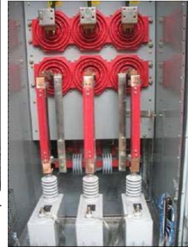
13.8kV snubber in metal enclosed switchgear
