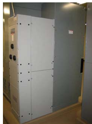
15kV snubber (compact) next to MV switch to transformer
