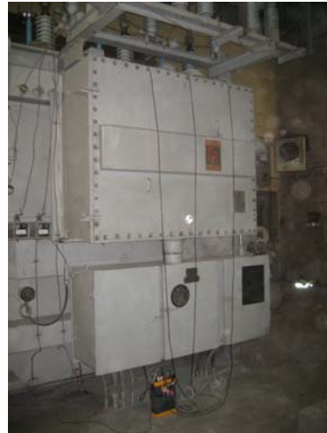
PQ Meter and Test Leads
