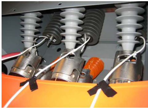
Fig. 21. Voltage divider connections at 18-kV surge arrester on transformer primary bushing.
