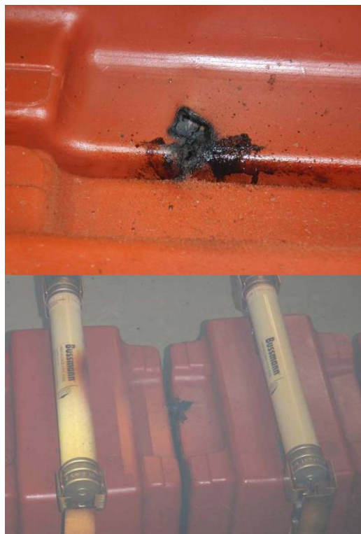
Fig. 1. Damage to PT but fuses remained intact.
