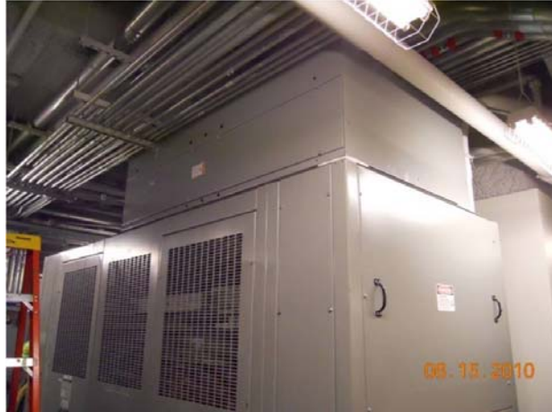
12.47kV snubber mounted horizontally above transformer 78" L x 45" W x 24" H
