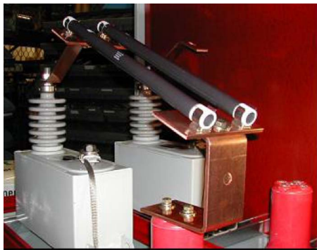
Fig. 15. 15-kV snubber mounted above the transformer.
