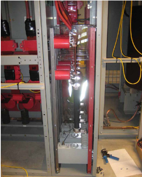
Fig. 15. RC snubber (typical installation for this facility).
