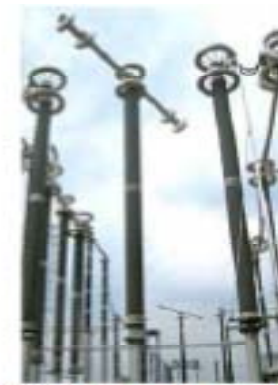
800kV DC Bypass Disconnect
