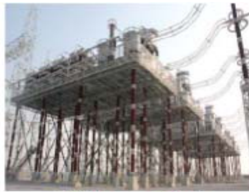
1100kV Series-capacitor bank
