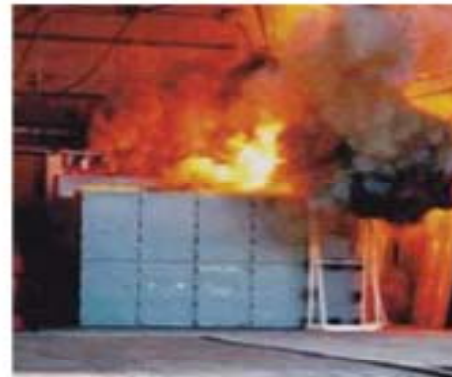
Internal arc failure
