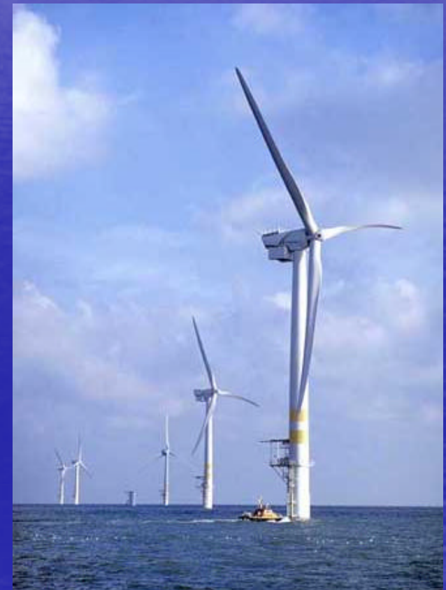
GE 3.6 MW Turbines Arklow Bank, Ireland
