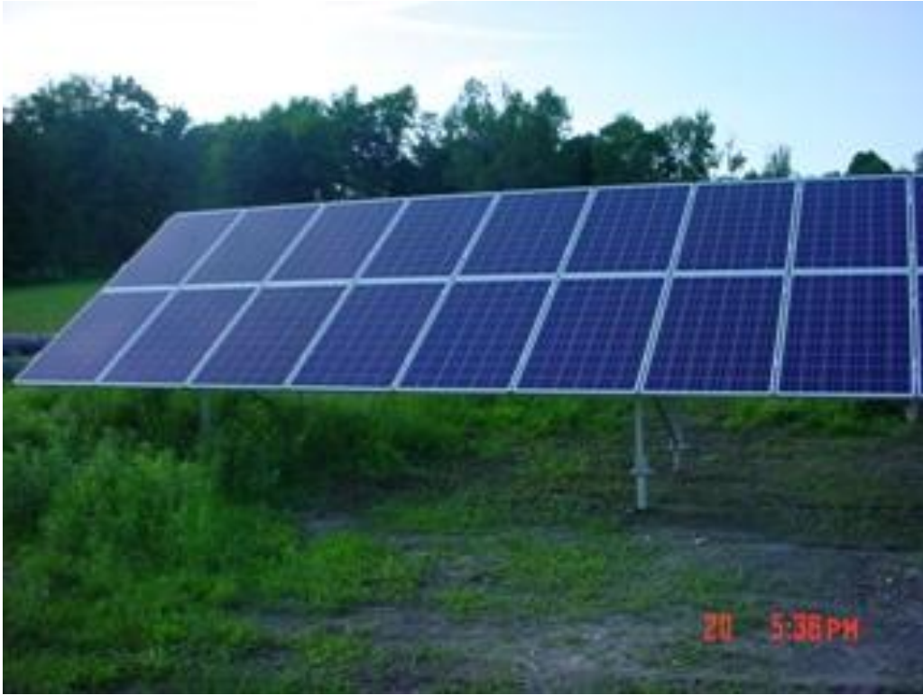
Roger's solar electric power system in operation – View 2
