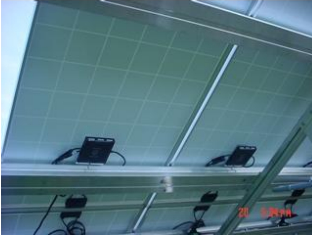
View of the microinverters converting 30 V DC to 240 V AC Single Phase, 60 Hz Power, one for each panel
