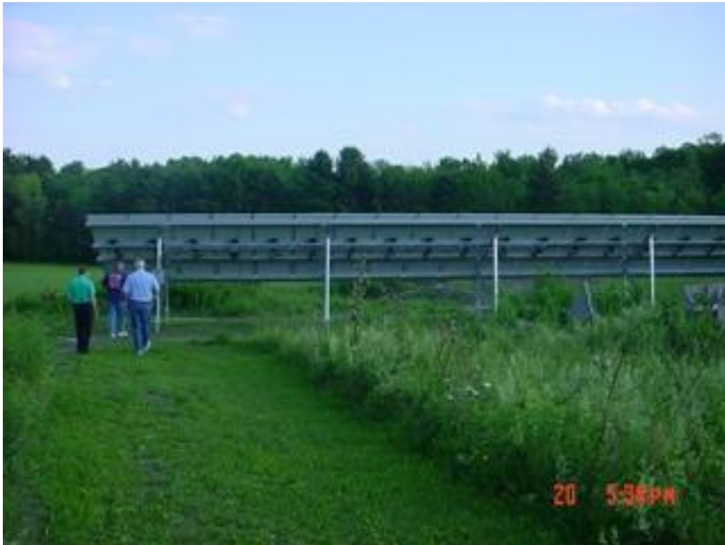
Roger's solar electric power system in operation – Back View
