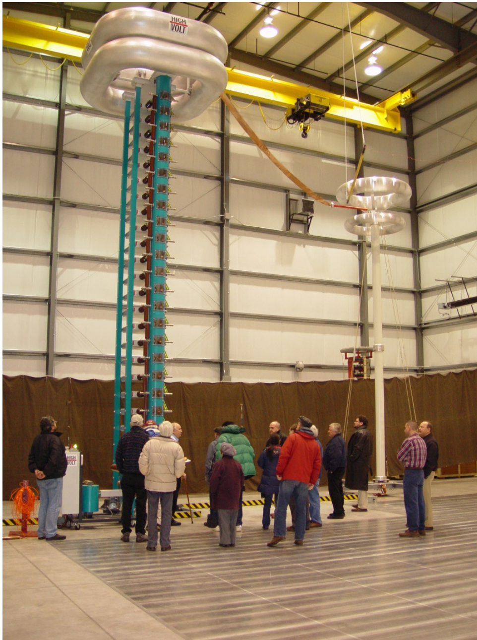
2400 kV Marx Generator at Lightning Technology, Inc.
