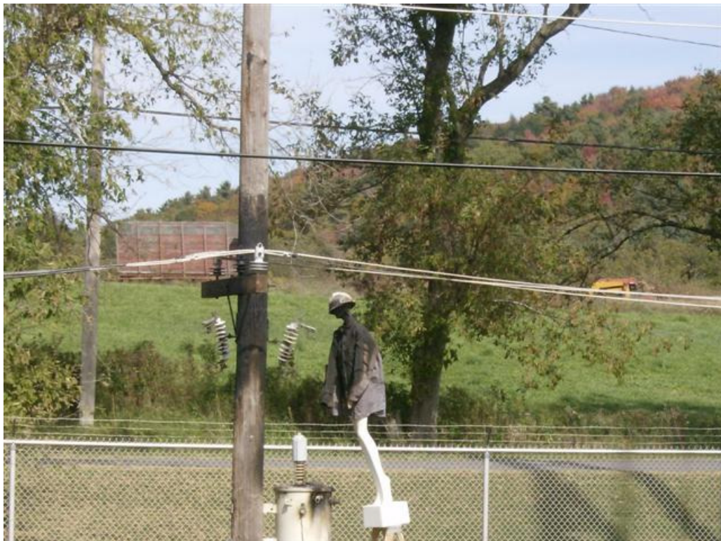
Figure 8 Aftermath of Arc Flash shows burned area on "Joe the Lineman"
