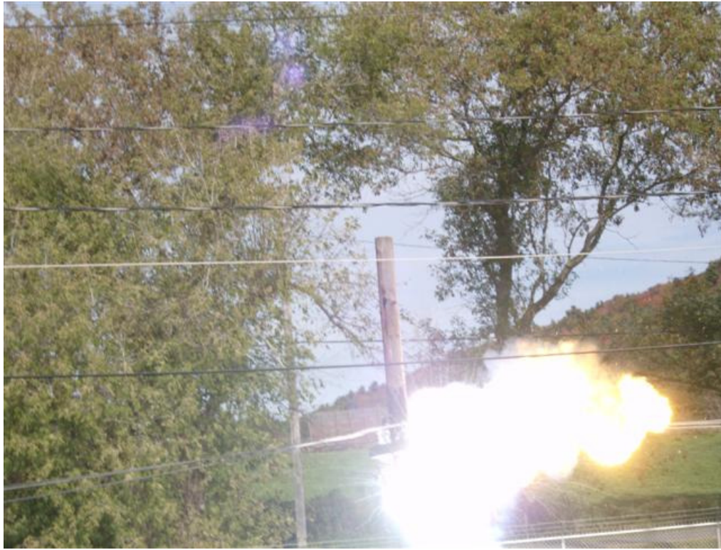
Figure 7 Arc Flash at 4000 to 5000 amps fault current. Note that arc flash engulfs "Joe the Lineman"
