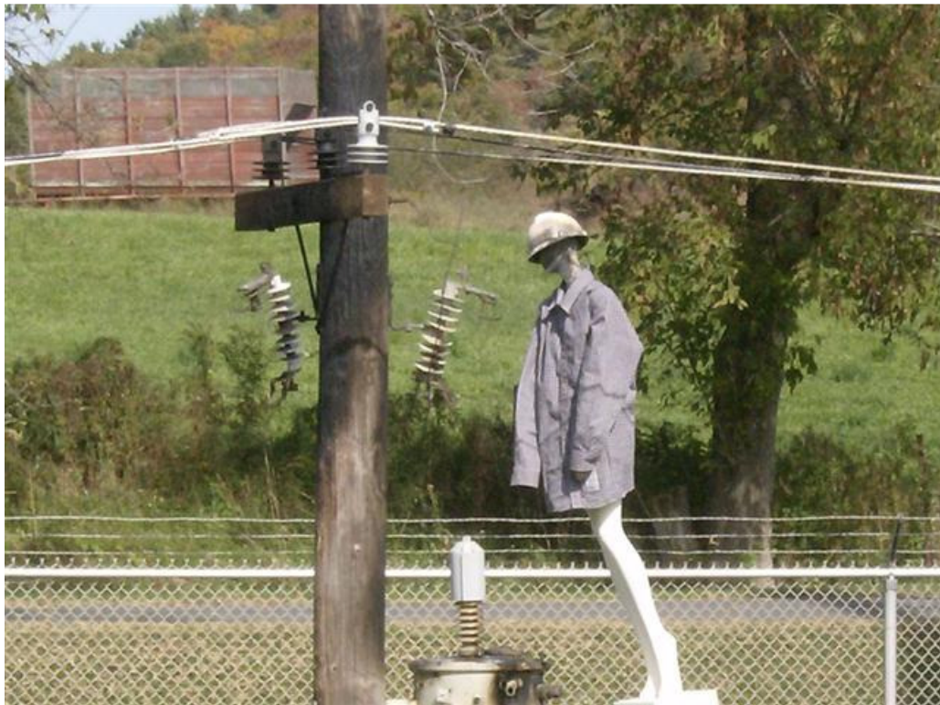
Figure 6 Close-up of fault arrangement. Outer phases are tied together with thin gauge solid copper wire to simulate fault. Outer phases are bonded to cut-out, as being worked on by "Joe the Lineman"
