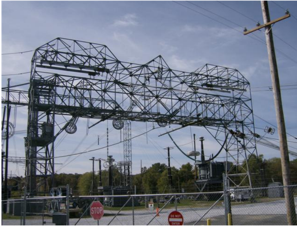
Figure 3 Tower 1 supports a 3-phase transmission line section with both horizontal and vertical adjustment
