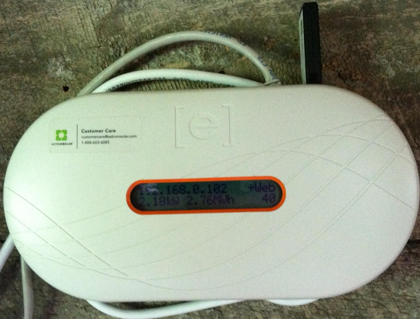
Envoy Communications Gateway in Garage
