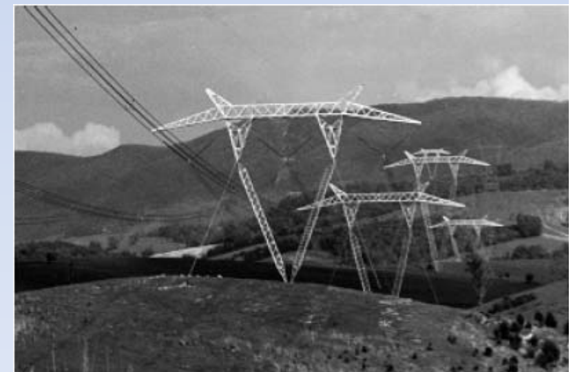
Figure 15.5-2 AEP 765-kV guyed-V suspension tower with four-conductor bundle.
