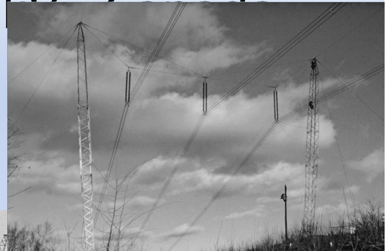
Figure 15.4-2 Hydro-Québec/TransÉnergie Chainette suspension tower.
