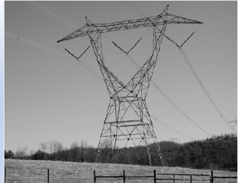
Figure 15.5-1 AEP 765-kV self-supporting suspension tower with four-conductor bundle.
