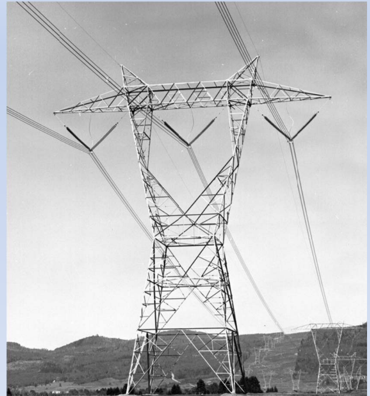
Figure 15.4-1 First-generation Hydro-Québec self supporting 735-kV tower.
