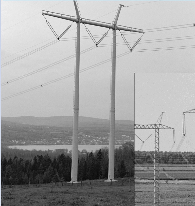
Figure 15.4-3 Hydro-Québec/TransÉnergie tubular self supporting tower.
