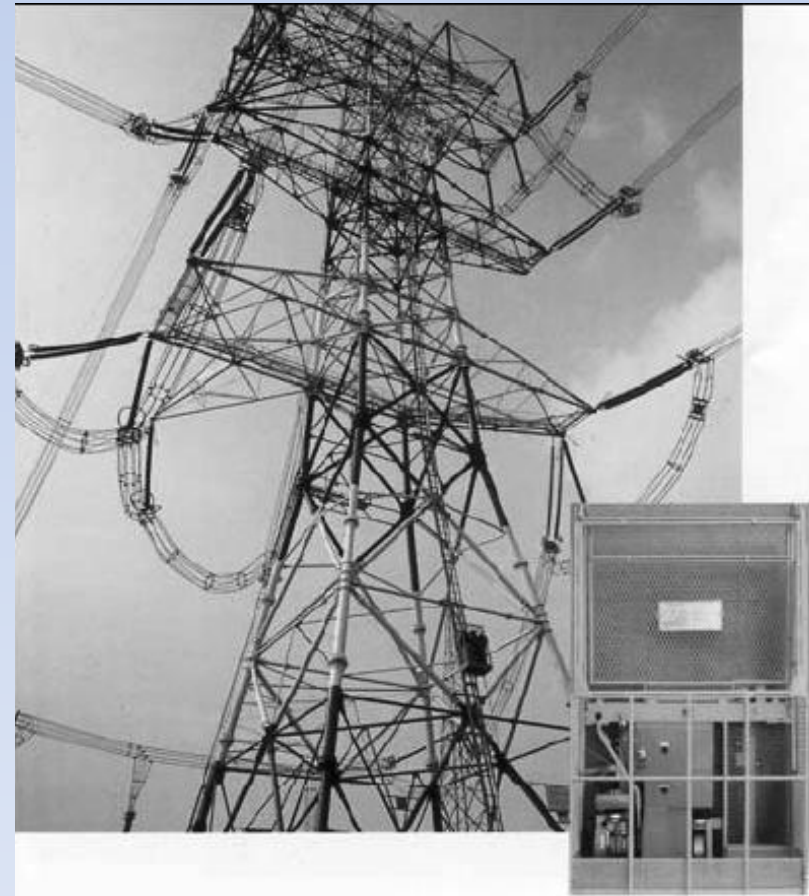
Figure 15.12-3 765-kV tower showing elevator and its rail.
