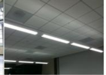
CA Lighting Tech Center UC Davis Campus Davis, CA
