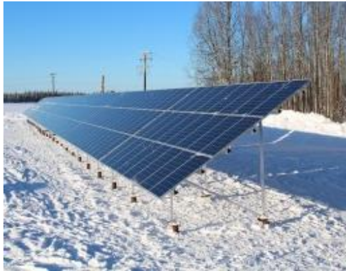
200 kW Bifacial Solar System
