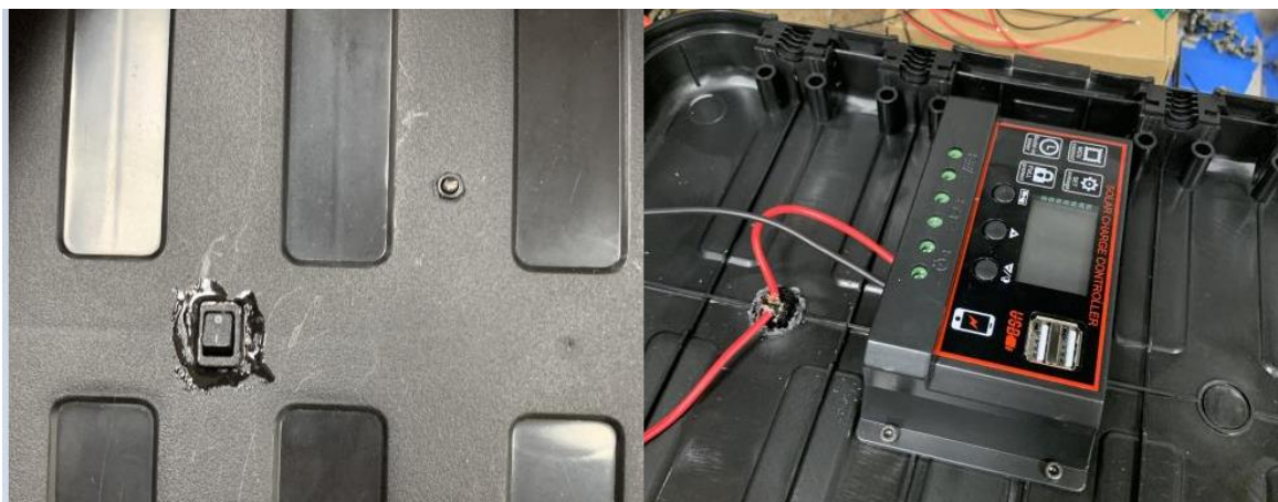
Figure 3.44 – SPDT Switch and PWM Charge Controller Installed to Lid
