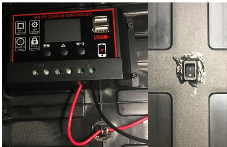
Figure 3.19 - Installation of PWM charge controller and ON/OFF switch in the lid of the control box.
