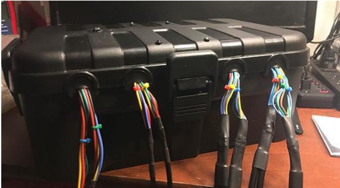
Figure 3.20 - Closed control box.
