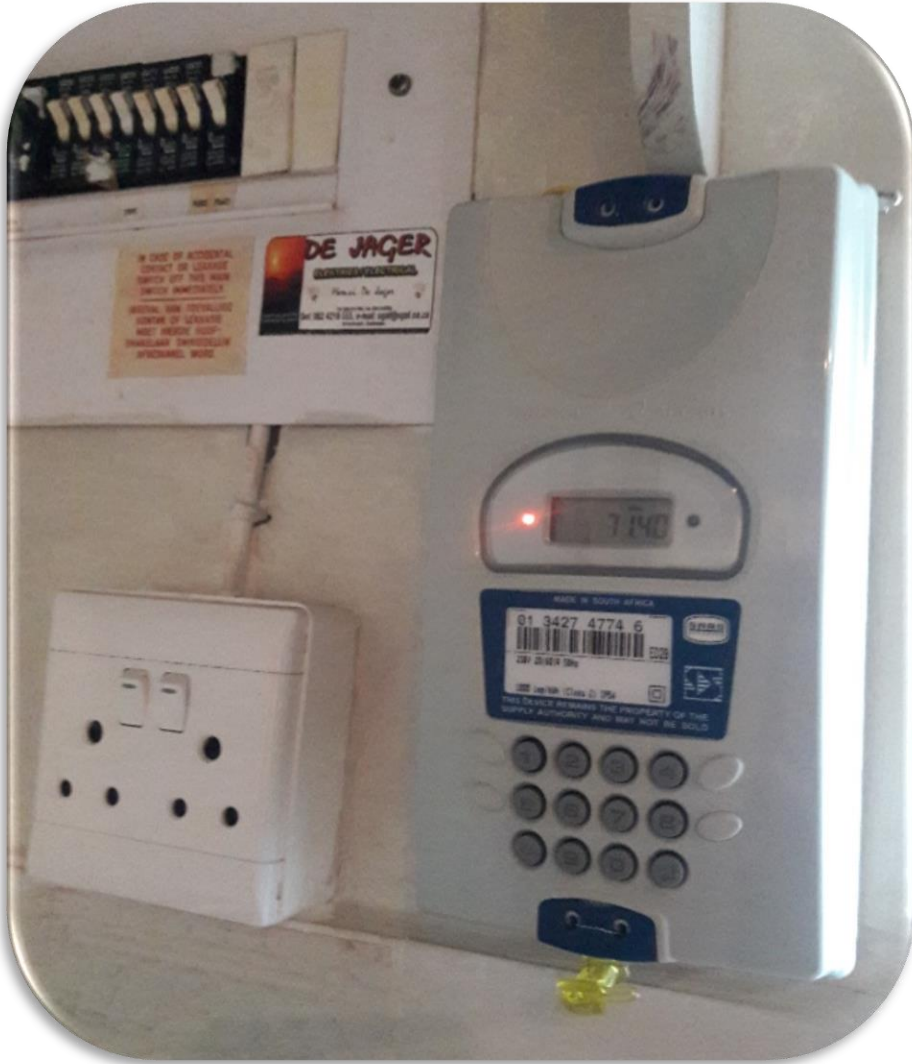
Prepaid Energy Meter
