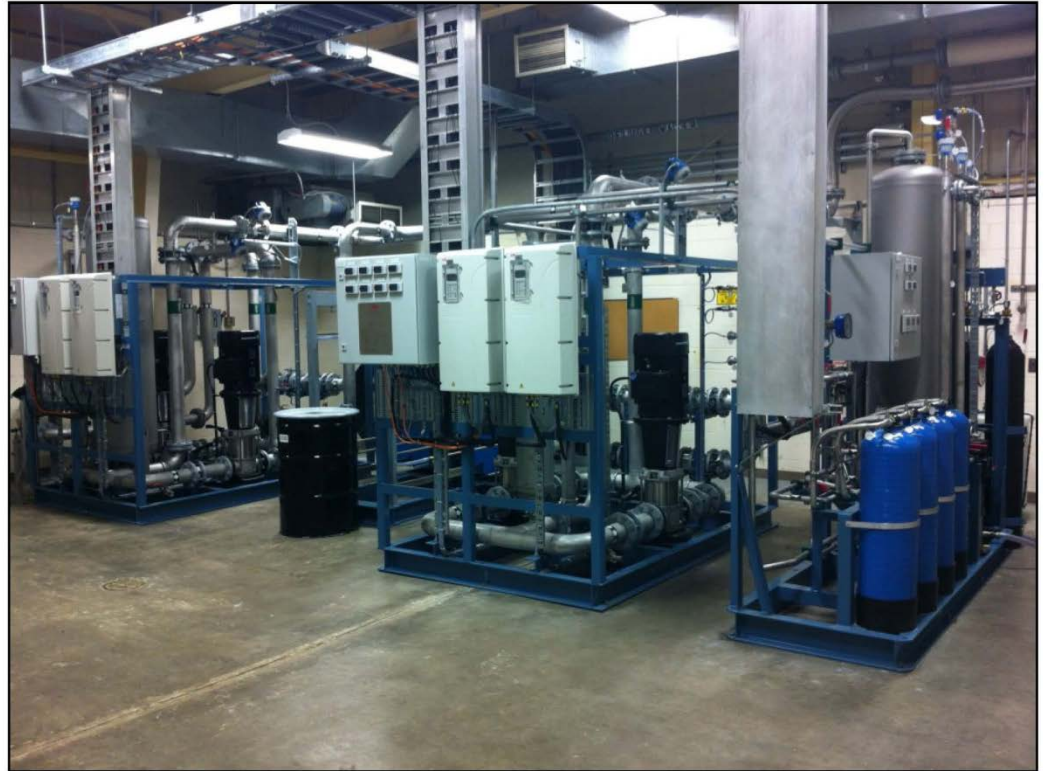
New Pump Cooling Equipment
