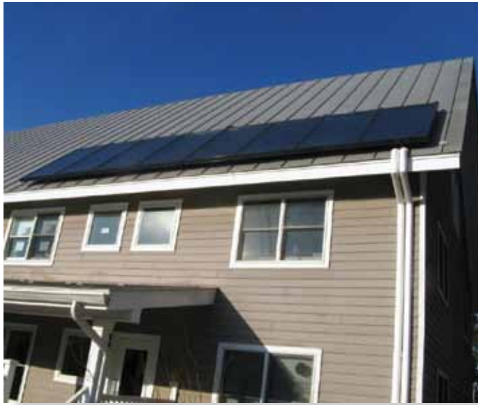
Students living in this residence hall at Bard College get most of their hot water from the sun, thanks to a new solar thermal system.
