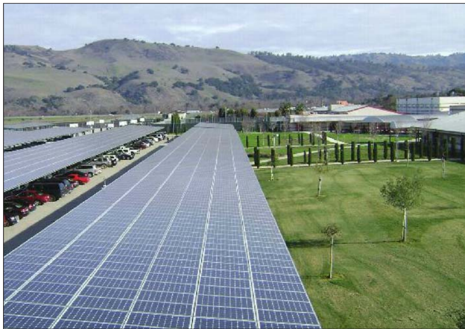
Solar panels shade the parking lot at Ann Sobrato High School in Morgan Hill.
