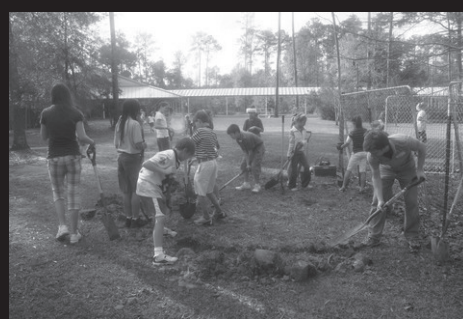
Figure 1. Students at an elementary school digging trenches to install their school’s plant nursery.
