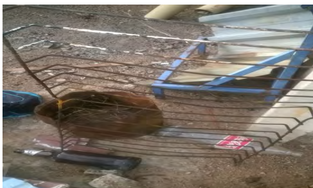
Rusted Iron Bars
