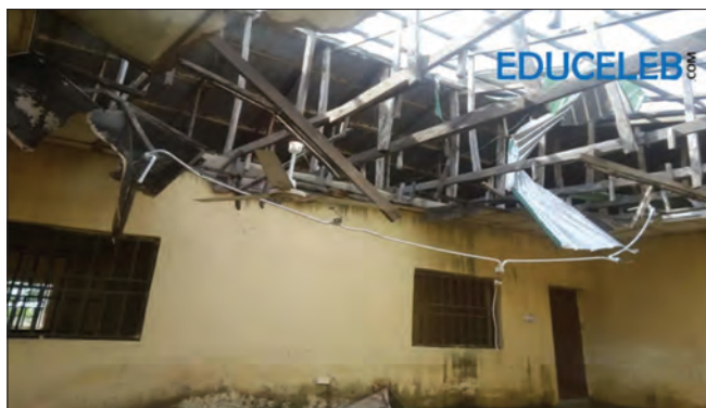
Figure 3: A dilapidated office within the administrative block of the Almajiri Model School, Dutsin-Ma. Source: Amoo (2019). Educeleb.com
