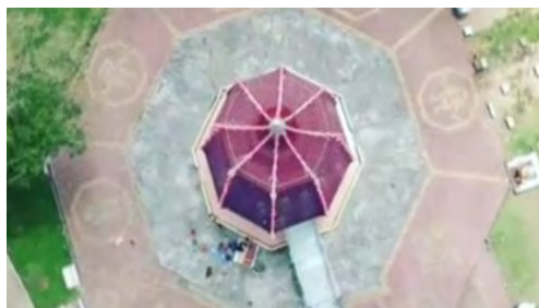
Pagoda Roof (Problem 1)
