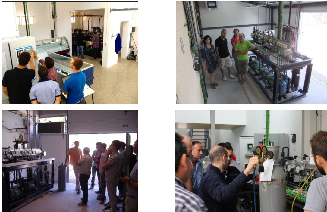
Figure 10. Launching of the cascade refrigeration systems. (Top-left: IES el Valle, Jaén; Top-right: IES Salvador Victoria, Monreal del Campo, Teruel; Bottom-left: IES Pou Clar, Ontinyent, Valencia; Bottom-right: IES Rascanya-Antonio Cañuelo, Valencia)
