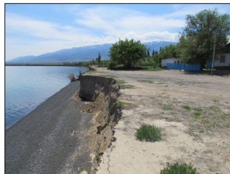
Figure 8. The destruction of the coasts near the village Koktuma (dangerous approach to the line of inhabited constructions)
