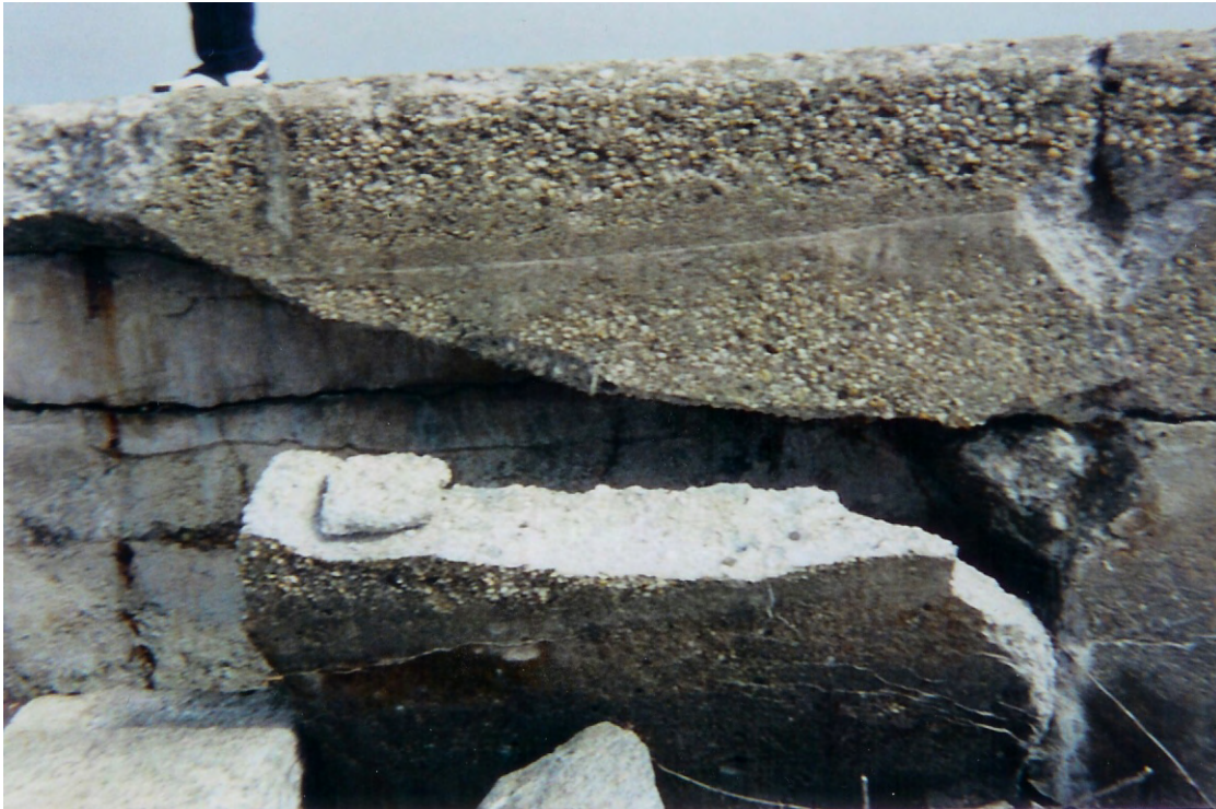
Figure 3. Student documentation of seawall erosion.
