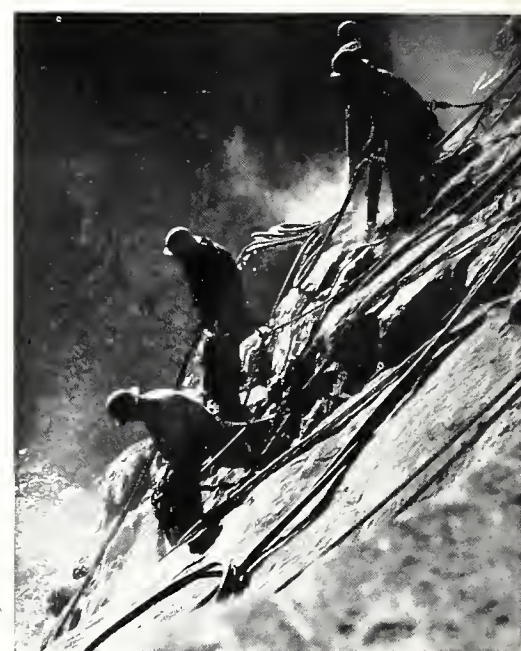
Drillers on Black Canyon Cliffs Preparatory to Construction of Boulder Dam. From Boulder Dam Film.
