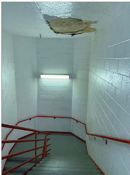
Ceiling damage from a roof leak in a New Mexico school.
