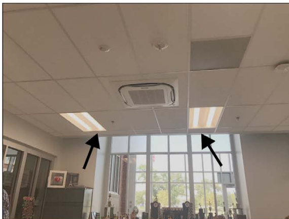
Light emitting diode (LED) lighting in a Maryland school
