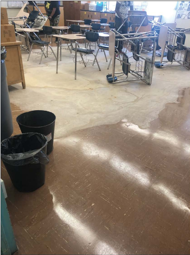
Water damage from HVAC leak in a California school, whose officials said replacing flooring is difficult because of asbestos floor tiles.
