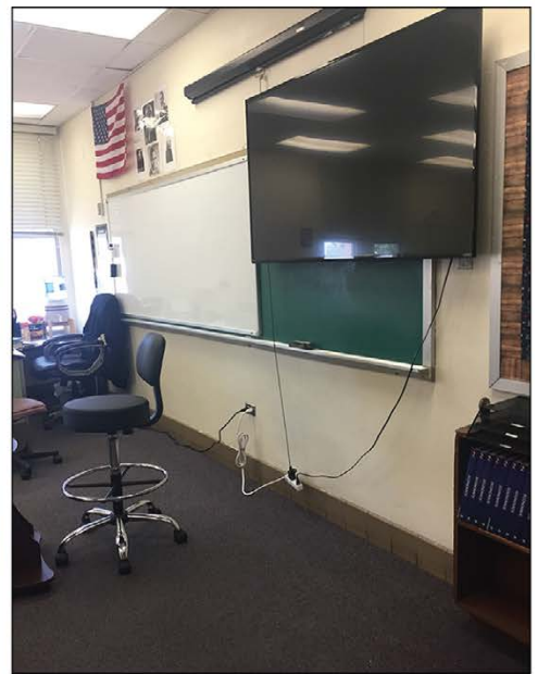
White board and screen placed on top of an old chalkboard so as to not disturb asbestos in the wall in a school in Florida.
