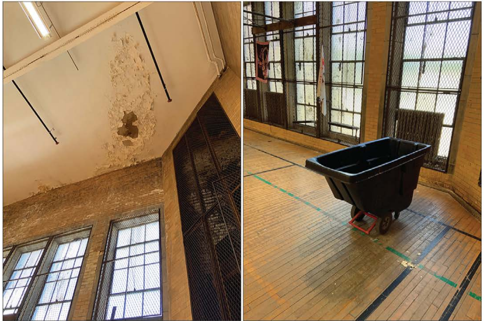
Roof leak in a Rhode Island school gym and bin underneath used to catch the water.
