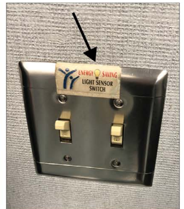
Lights in a California school automatically turn off when rooms are not in use
