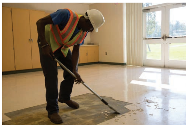
Brewster Middle School classroom repair after hurricane Florence
