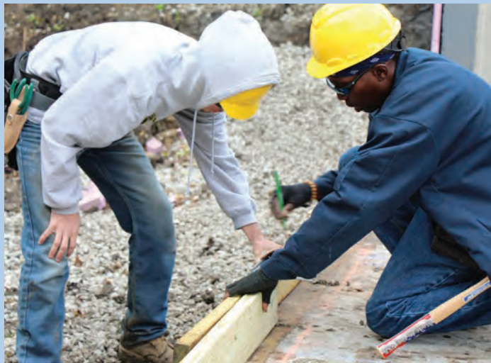
Students in Southwestern's high school and college carpentry and building trades programs build affordable housing for the region
