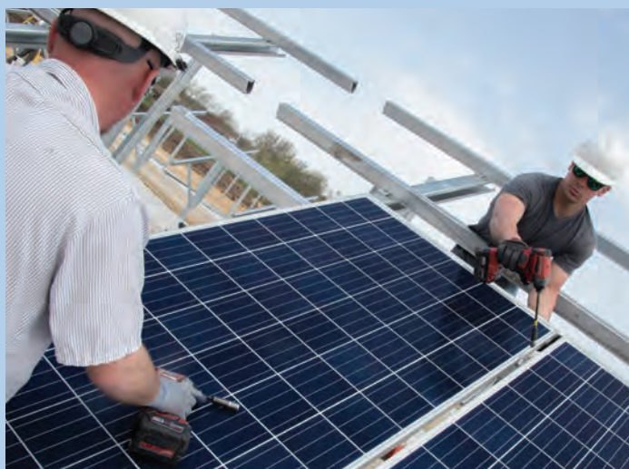
Solar panels at Southeastern Community College's Keokuk campus
