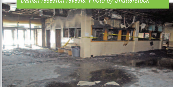
North Dakota. The inside of Trinity High School shows heavy damage from a fire. The entire school has visible and extensive smoke and water damage from the blaze in the office area. Photo by Tom Stromme/Bismarck Tribune
