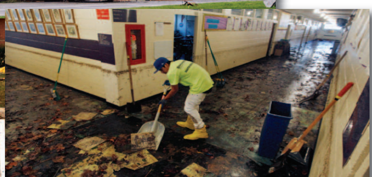
New Jersey. School damage after Hurricane Sandy. Photo by Rich Schultz
