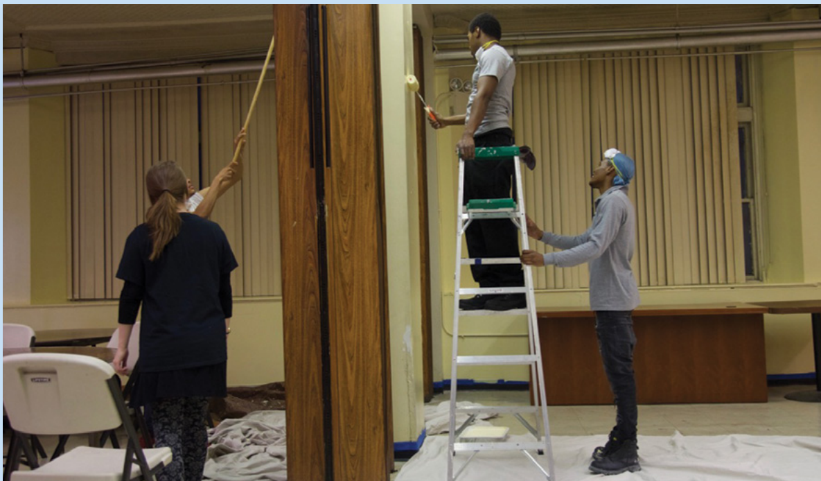
Harlem Justice Corps members painted the community room at All Souls' Episcopal Church.
