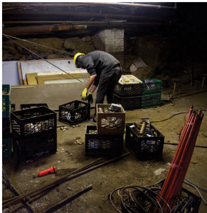
Bronx Justice Corps member clearing the New Covenant Gospel Temple basement, which will house a vocational training classroom.
