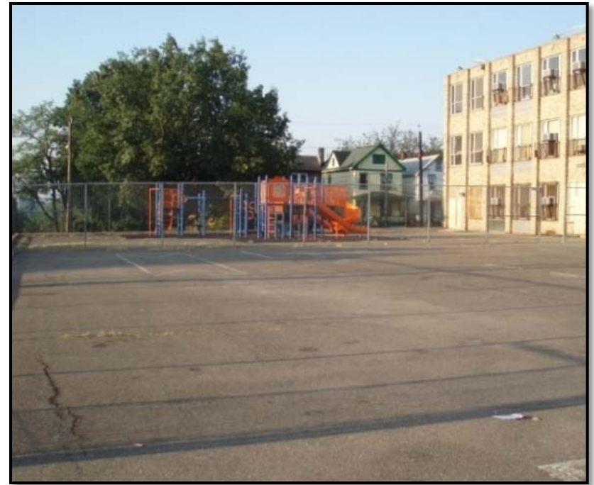
Poor Quality Hardscape with Old Equipment Martin Luther King Elementary School
