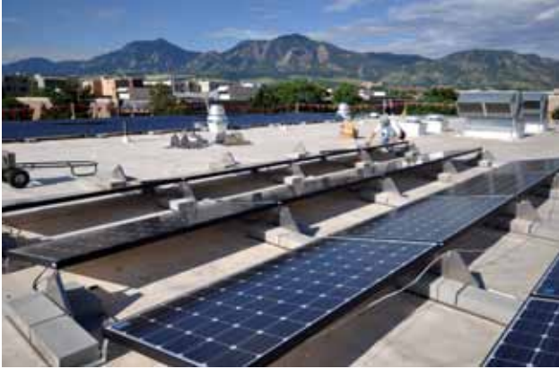
The photovoltaic panels pictured above are located on the roof of the Wolf Law Building, and are just 52 of the total 472 panels located around CU that help to offset campus-wide energy use.
