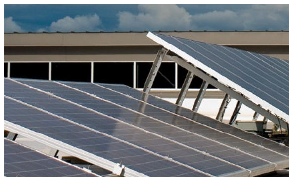
Three kilowatts of photovoltaic panels have been installed on the roof of a building at Lane Community College. These installations were funded by Lane's revolving fund and the Energy Trust of Oregon.
