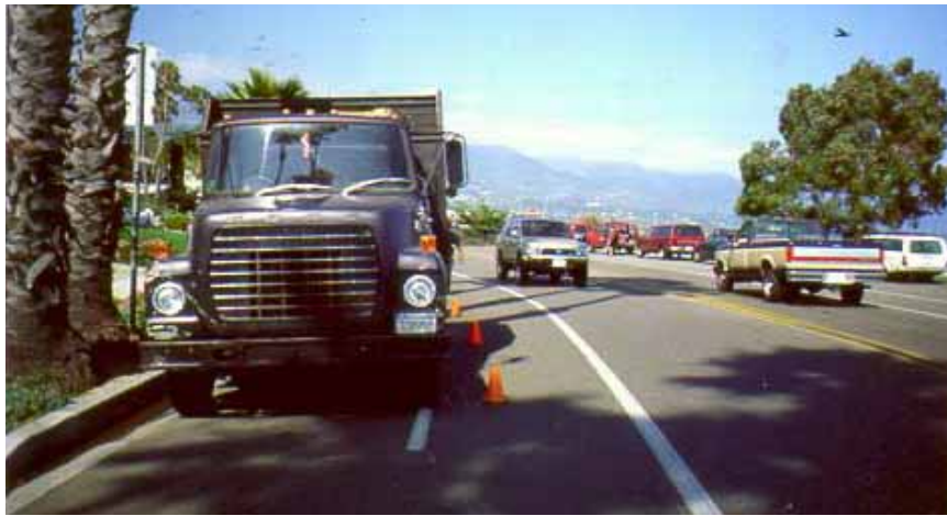
Figure 21-1. Utility work in bike lanes can often be accomplished without blocking the entire lane.
