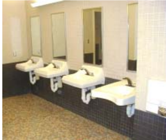
Rough service grade fluorescent lights, like the ones over these mirrors, last long, continue to look good, and do not suffer from cracks and other signs of abuse.
