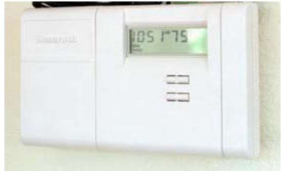
Adjustable thermostats allow the user to have control over the conditions of the room, which can improve overall comfort and create a better learning environment.
