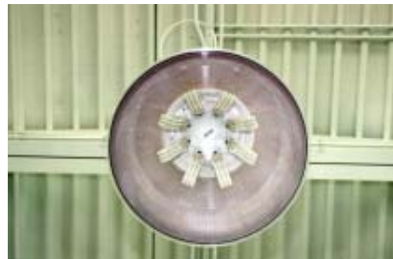
Compact fluorescent lighting fixture. NREL/PIX 09211
