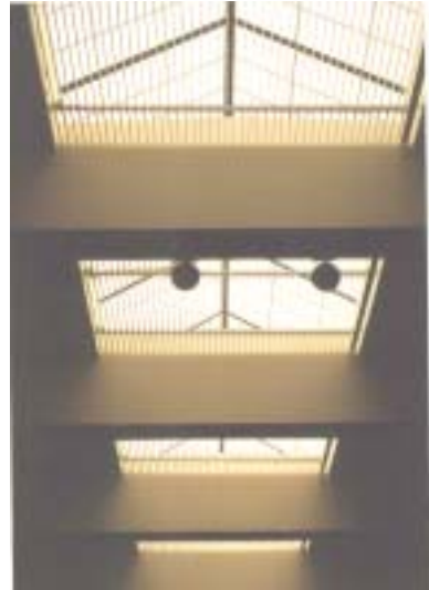
Linear skylight in multipurpose room includes electrically operated louvers to reduce brightness when needed.
