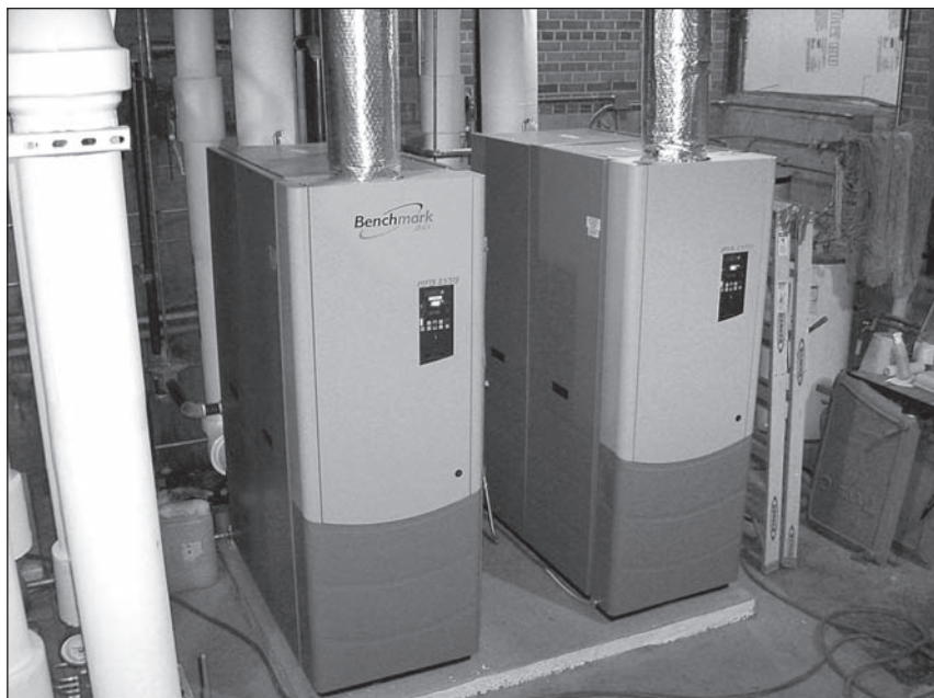
High school's recently installed heating system
