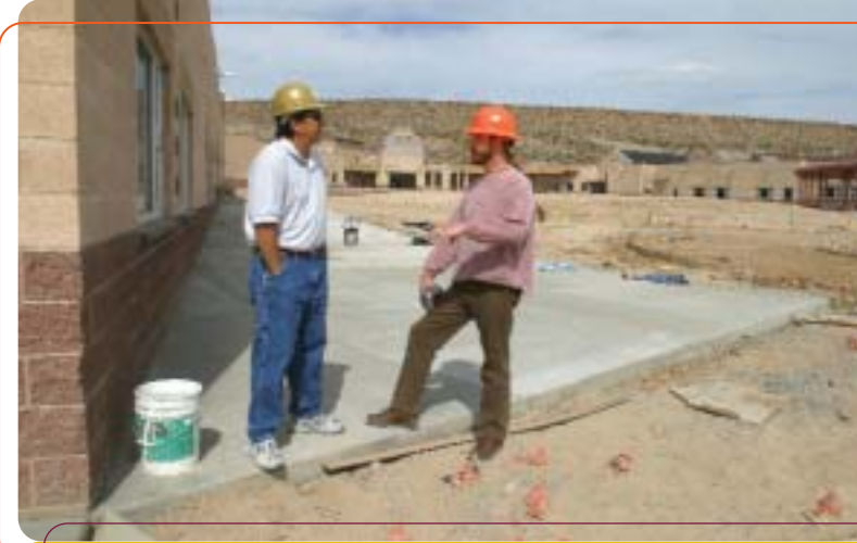
Mark Thompson, KLCC Fellow and project manager for the new Laguna Acoma High School, and Phil Sittnick, KLCC program coordinator, taking a tour of the school's progress.
