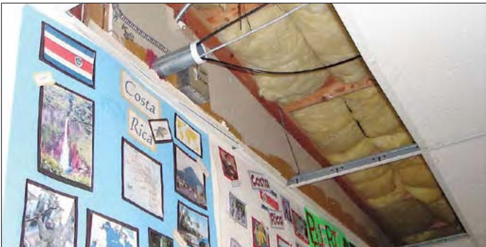
Damaged ceiling tiles were removed in this California classroom, exposing students to electrical wiring and insulation fibers.
