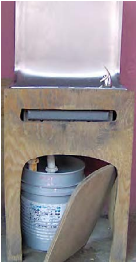
Water efficiency is a key element of sustainable design, sorely lacking in this Virgin Islands school.
