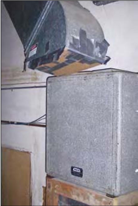
HVAC systems in many schools are in a bad state of disrepair.
