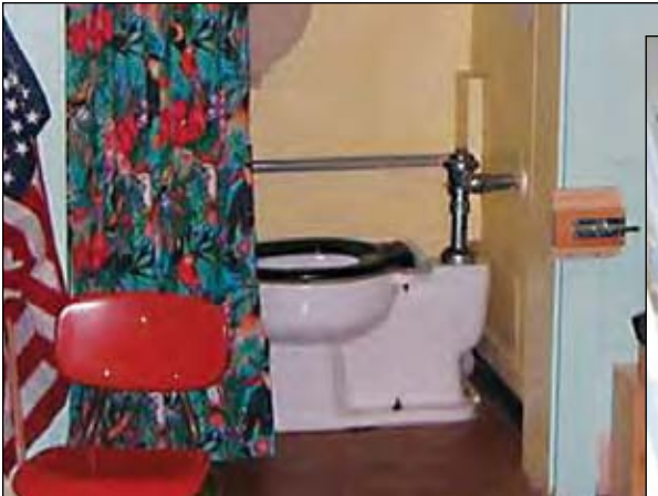
Before: Only a thin curtain separated this bathroom from the classroom.
