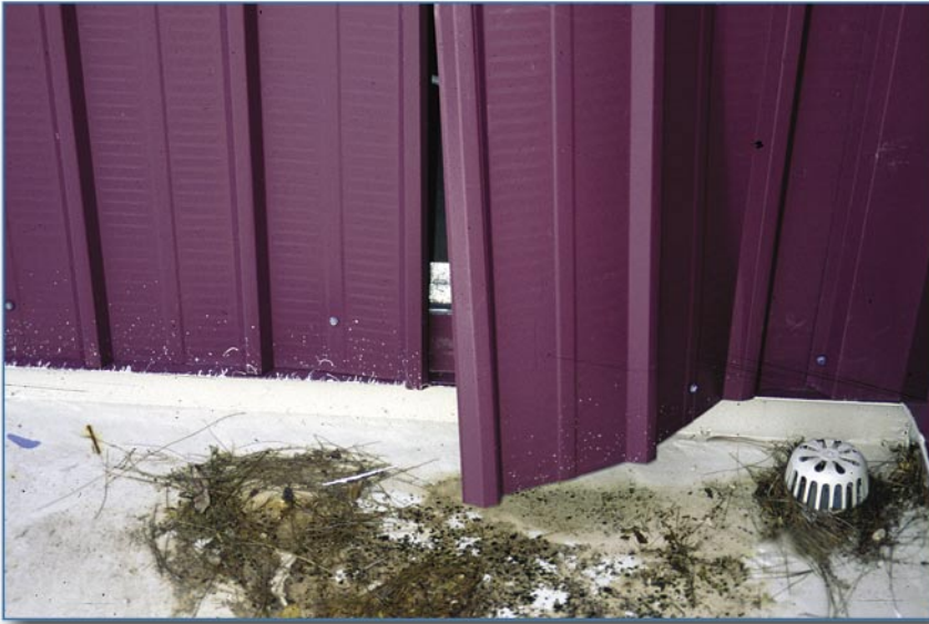
Figure 6-43 The parapet on this school was sheathed with metal wall panels. The panels were fastened at 2 feet on center along their bottom edge, which was inadequate to resist the wind load.
