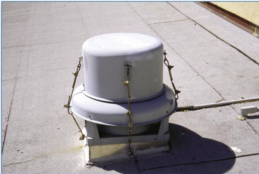
Figure 6-51 To overcome blow-off of the fan cowling, which is a common problem, this cowling was attached to the curb with cables. The curb needs to be adequately attached to carry the wind load exerted on the fan.
