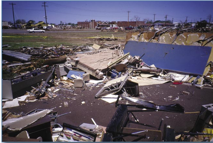
Figure 6-15 The roof and all the walls of a wing of this elementary school were blown away by a violent tornado.
