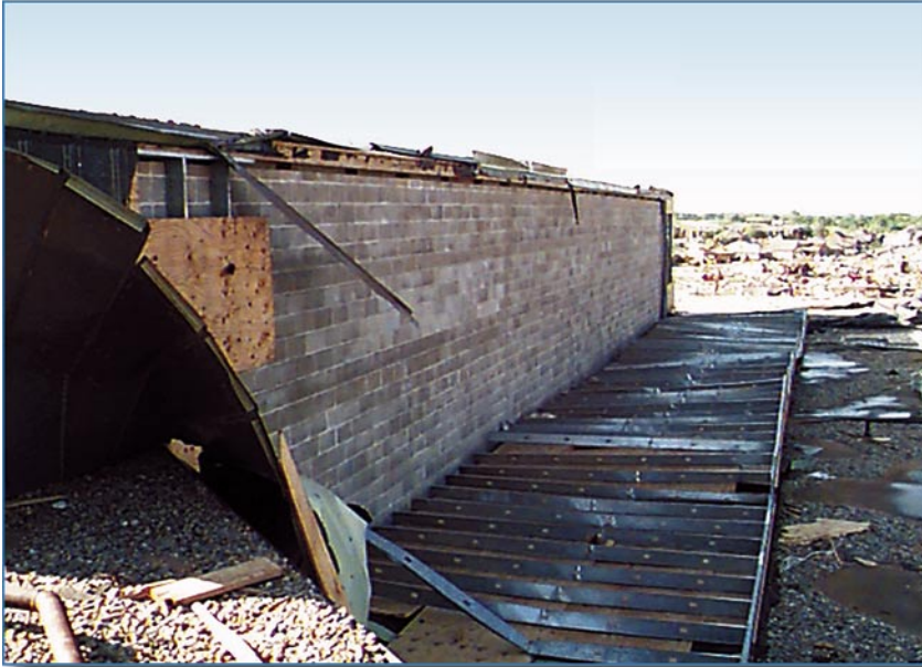
Figure 6-13 The metal wall covering on this school was applied to plywood over metal studs. The metal stud wall collapsed in this area, but, in other areas, it was blown completely away. The CMU wall behind the studs did not appear to be damaged. This school was on the periphery of a violent tornado.
