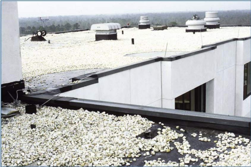
Figure 6-8 The aggregate ballast on this single-ply membrane roof was blown away in the vicinity of the corners of the wall projections at the window bays. The irregular wall surface created turbulence, which led to wind speed-up and loss of aggregate in the turbulent flow areas.
