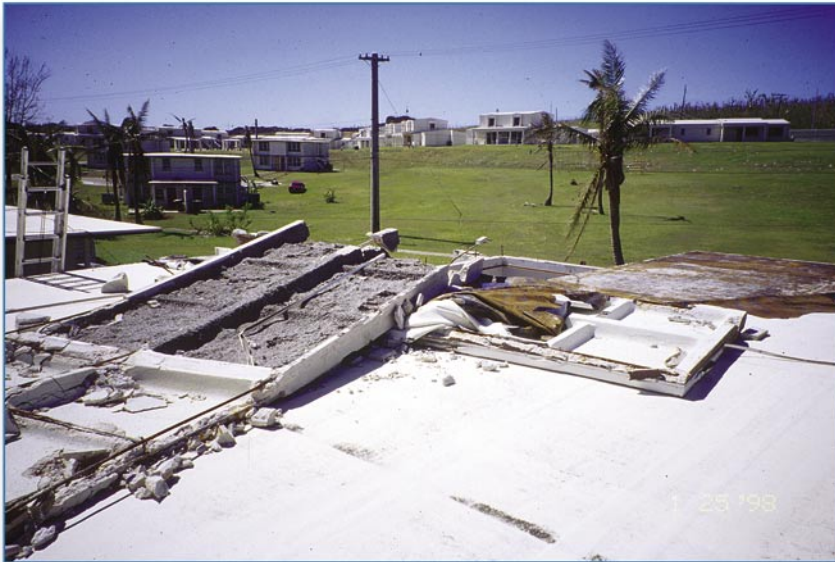
Figure 6-23 Portions of this waffled precast concrete roof deck were blown off. Bolts had been installed to provide uplift resistance; however, anchor plates and nuts had not been installed. Without the anchor plates, the dead load of the deck was inadequate to resist the wind uplift load.
