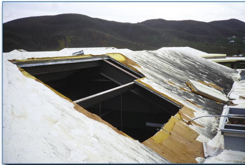
Figure 6-58 This school had a cementitious wood-fiber deck (commonly referred to by the proprietary name “Tectum”).
