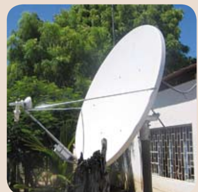
Satellite dish installed at the Institut Halieutique et des Sciences Marines in Tulear, Madagascar, to facilitate VSAT Internet access. The Very Small Aperture Terminal is a ground station used to communicate data via satellite.
