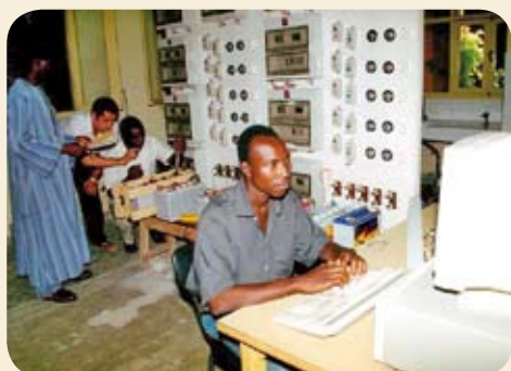
Sizing of a solar system and simulation of an electric breakdown during practical training organized within the solar summer school in 2001.
