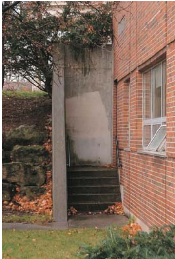
Partially hidden entryways can provide opportunity for would-be vandals.
