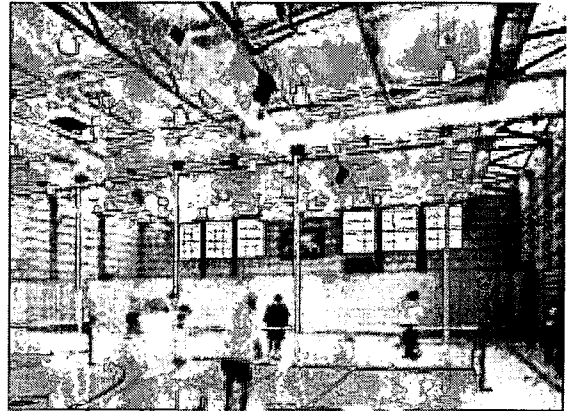
Metal halide gym lighting. Windsor High School Gym, Photo courtesy Quattrocchi / Kwok Architects
