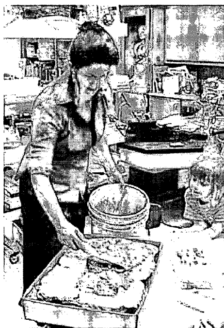
Ms. Berry used concrete brought in by the brick masons to smooth a mud slab on top of the grade beams the students had poured the previous week.
