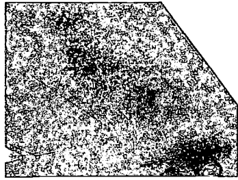
Water stained ceiling tile in Room 13 of Building 624.
