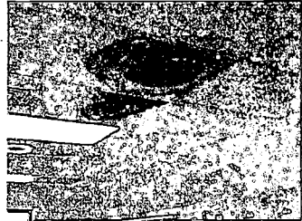
Ceiling tile damaged in hall corridor of Building 626. Note that water has also leaked into light fixtures.
