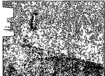
Wall of Building 626 shows damages caused by water. The light areas are where patches have been made.
