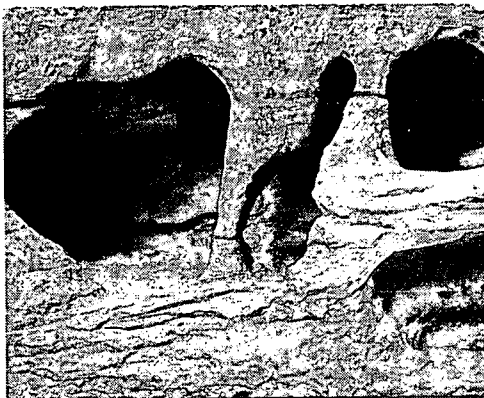
weathering caused by water
